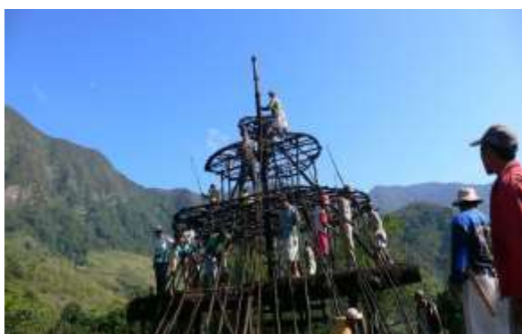
Gambar 11, 12, 13: Proses restorasi Mbaru Niang di Desa Waerebo, Flores (Sumber: https://bandanaku.wordpress.com , diakses 08 Mei 2017)
