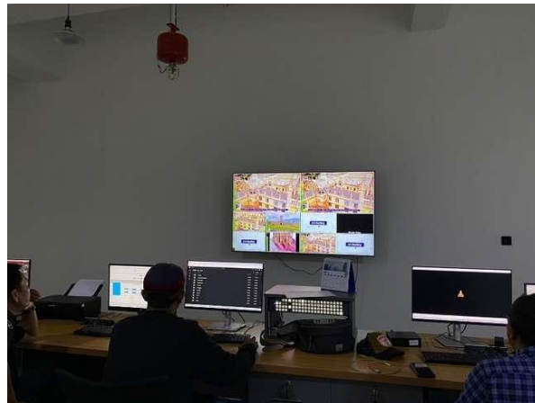
Gambar 4. 14 Master Control Room
